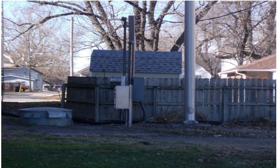
Above-ground equipment for existing Sanitary Sewer System Pump Station adjacent to residential property to the west including privacy fence, storage shed, and single-family residence. (Pump station telemetry antenna located atop stainless steel pole on right.)
